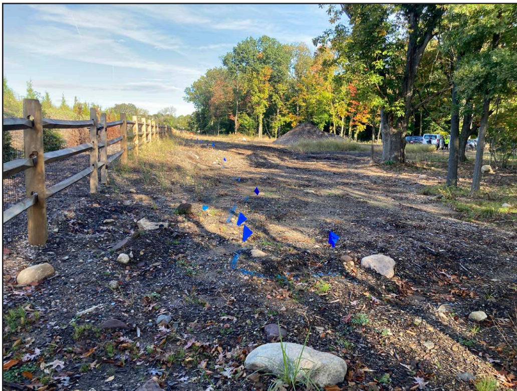
Plate 4.12: View along the Route 17 corridor showing the installed fencing, earth and stone berm, and subsurface water utility pipeline.
