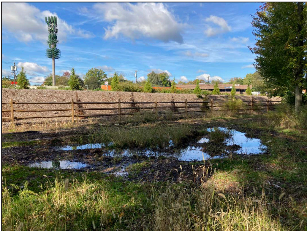
Plate 4.20: Standing water within the graded areas along the Route 17 corridor.
